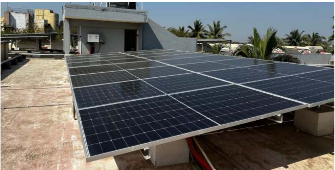
Picture 1 : Solar Panels installed at the Hanumat hospital
